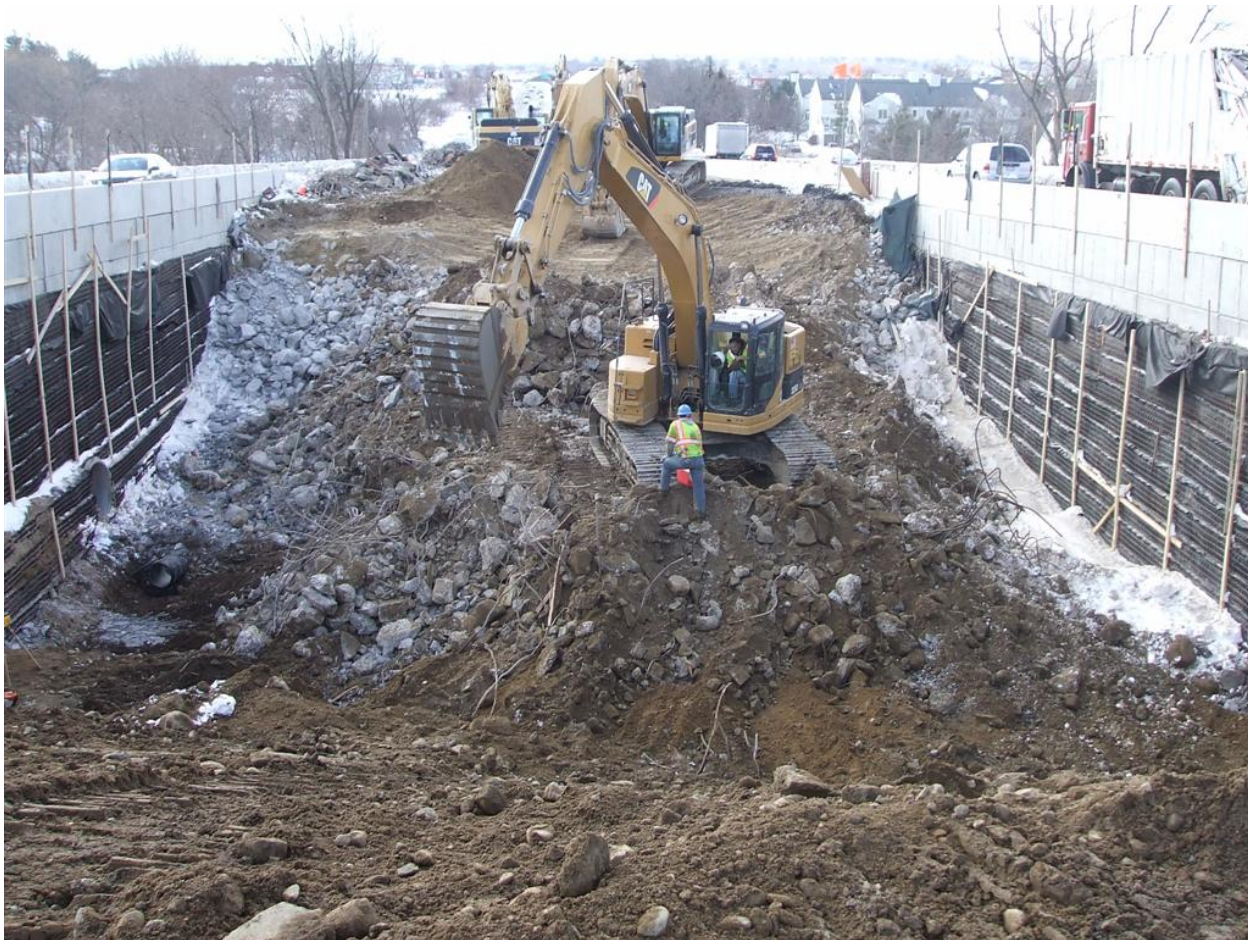
Area of existing bridge (Route 128 over the Railroad Corridor) that has been demolished. Photo also shows temporary Mechanically Stabilized Earth (MSE) walls constructed on either side of the existing bridge to support temporary Route 128 travel lanes.
